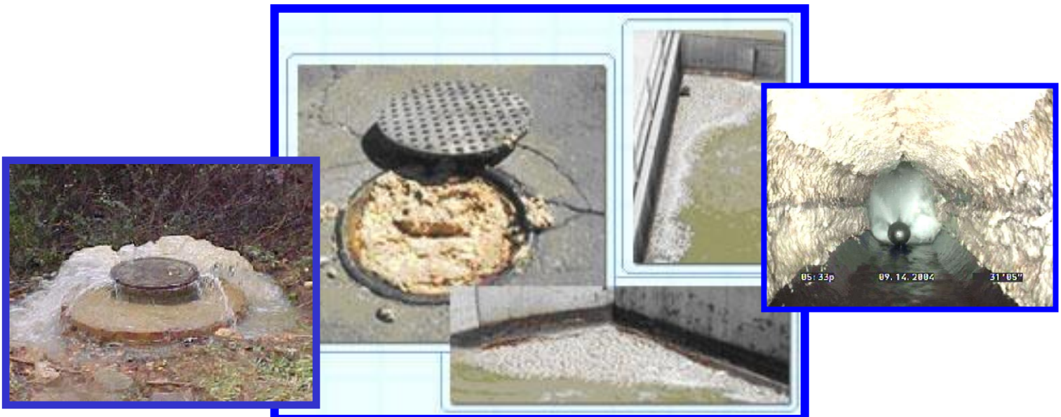
Figure: The effects of FOG accumulation in the sanitary sewer system.
