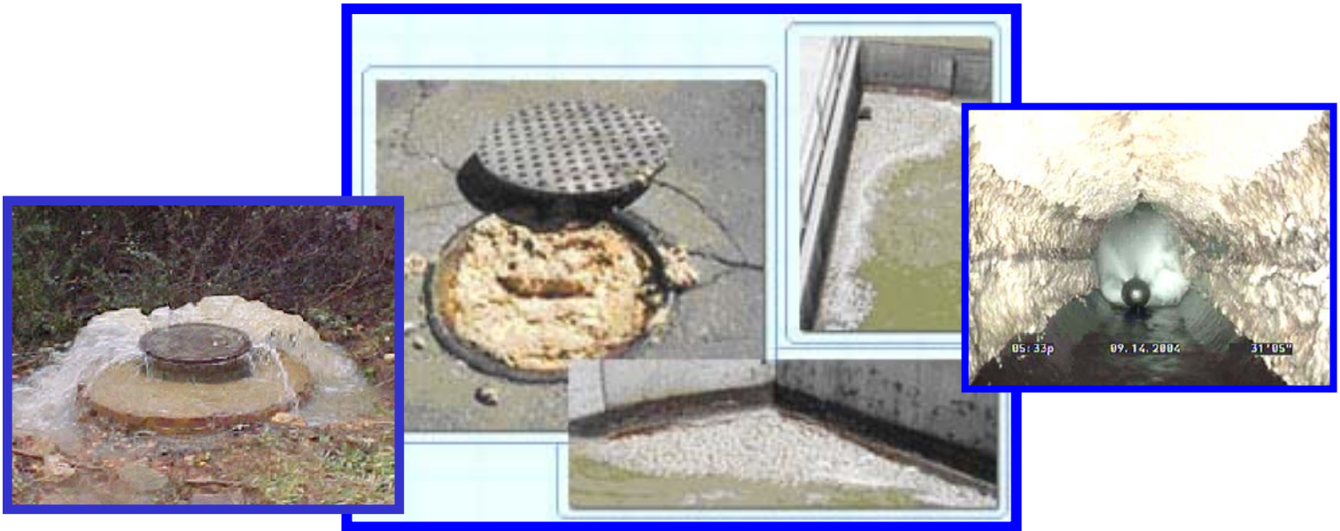
Figure: The effects of FOG accumulation in the sanitary sewer system.
